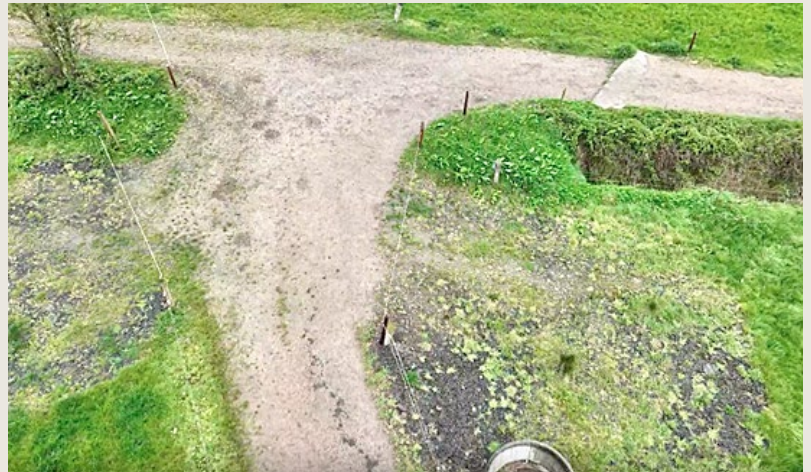
Pictured above: A crossing point that was widened with the widened parts covered in topsoil and grass seed.
