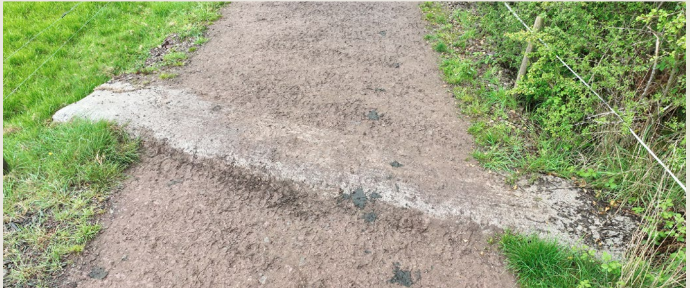
Pictured above: A concrete bar diverts water off the farm road to reduce risk of pollution to a watercourse. Note how it extends into the field to avoid streams channelling around it.
